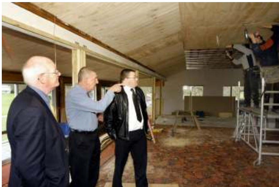
President Alan Jamieson, project manager Graham Curgenvin and Eureka Trust CEO Graeme Parker inspect the renovation work being done on the pavilion.
